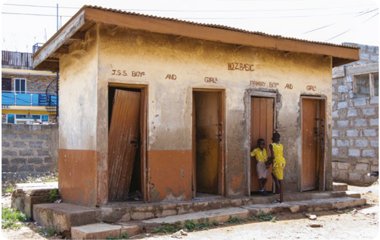
A Typical old-fashioned sub-standard school toilet.
